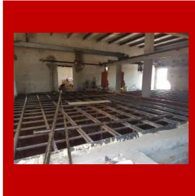
Automatic Block Ice Plant
